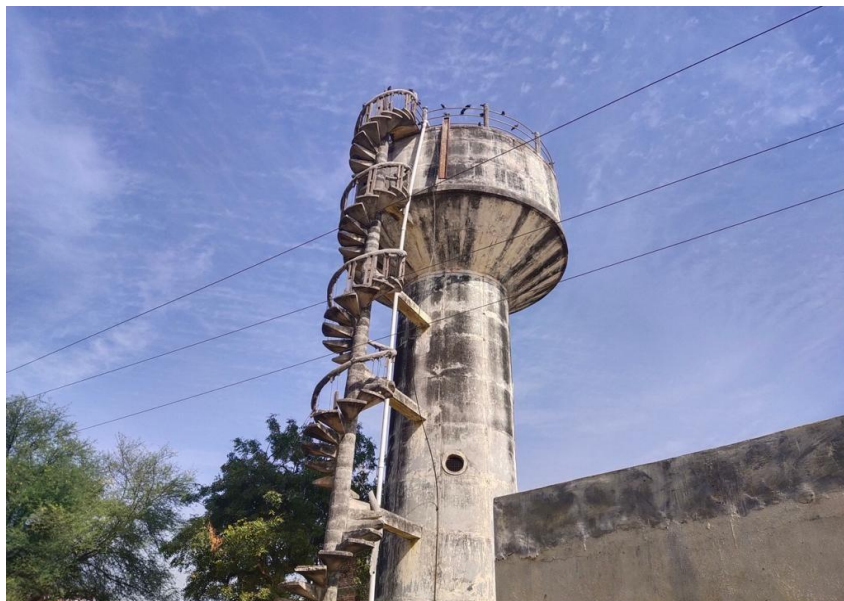
Over head water tanks
